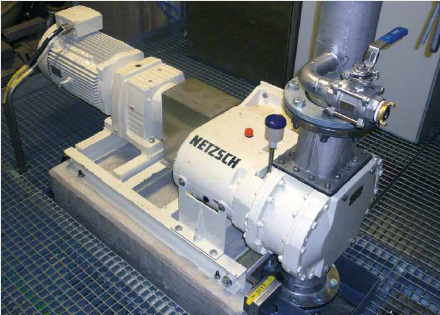
A TORNADO® pump in a paper factory for unloading Kaolin from tankers. Flow rate is 75 m 3 /h and pressure is 4 bar.
