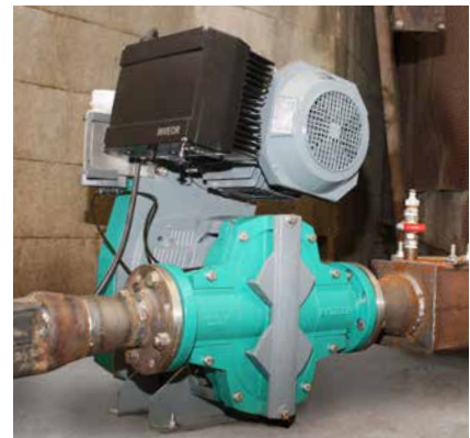
Pumping liquid manure in a biogas plant
