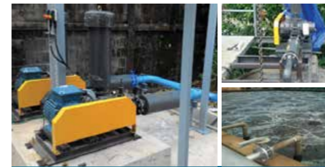
1. Water Treatment System
