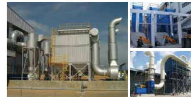
3. Dust Collector System
