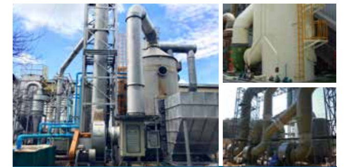
2. Wet Scrubber System
